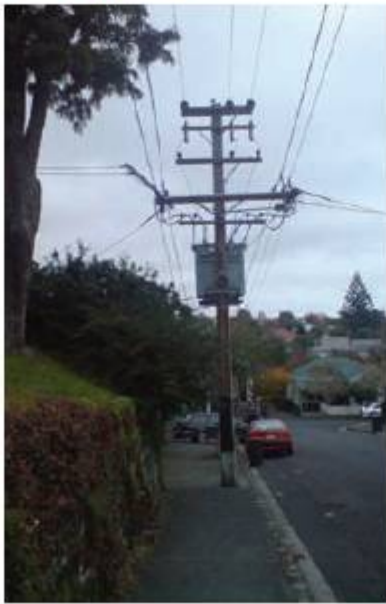
Figure 7.3 A transformer on a post supporting overhead power lines “steps down” the voltage used in power distribution lines to the 110/240V mains supply used by homes
